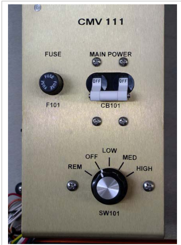
Figure 11a CMV-111 Control Module
